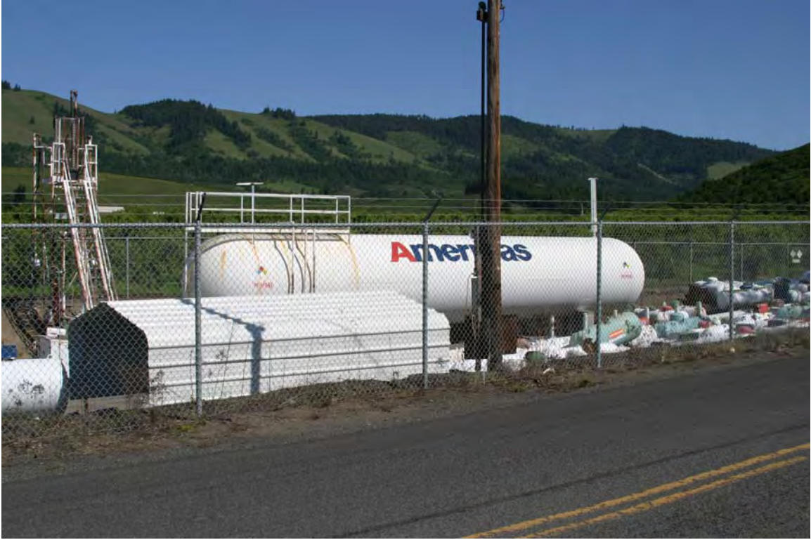
Figure 15: Propane Tanks in the Pine Grove District
